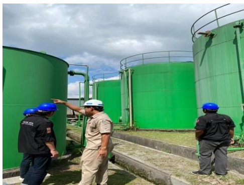
Gambar 3. Demineralized Water Storage Tank
