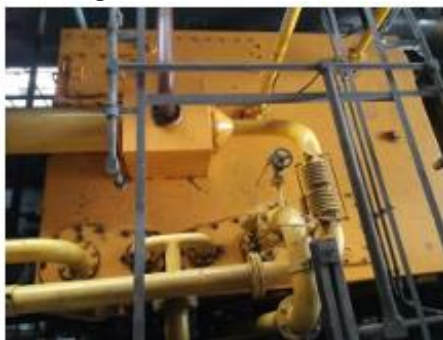
Gambar 2 Main oil tank
