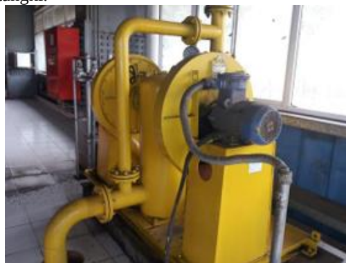
Gambar 11 Main oil tank Exhaust Fan
