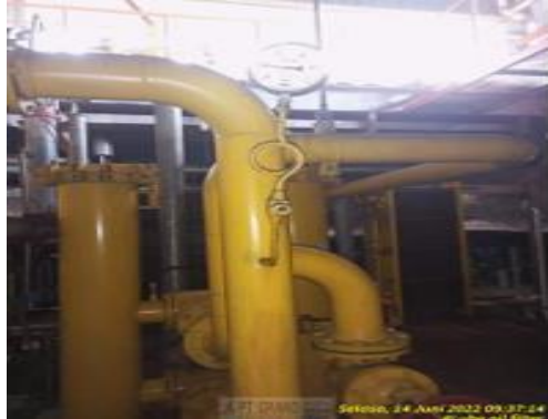
Gambar 7 Lube Oil Filter
