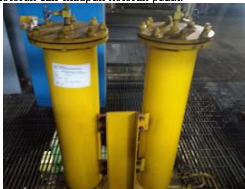
Gambar 8 Turbine Lube Oil Conditioner
