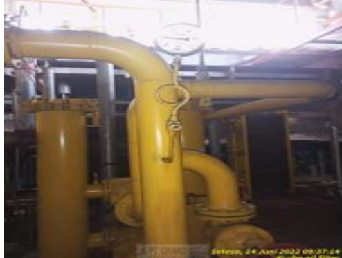
Gambar 7 Lube Oil Filter
