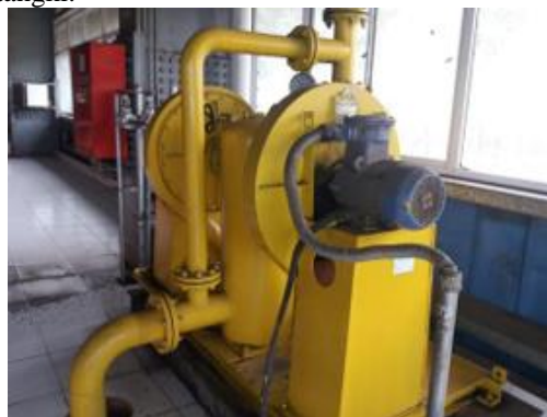
Gambar 11 Main oil tank Exhaust Fan
