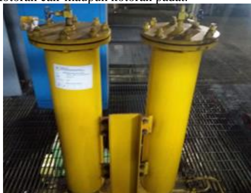
Gambar 8 Turbine Lube Oil Conditioner
