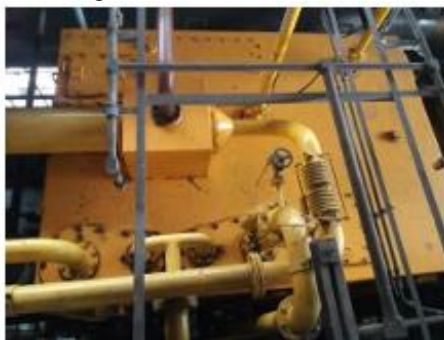
Gambar 2 Main oil tank
