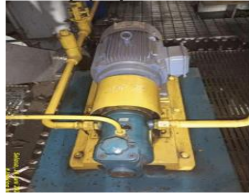
Gambar 9 Jacking Oil Pump
