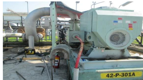
Gambar 4.1 Pompa 42-P-301 A
